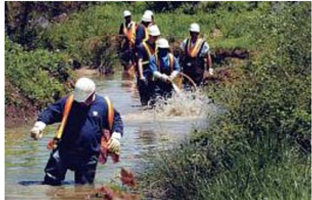
William Prevatt, an employee of the city of Raleigh, stirs muck from the bottom of Sycamore Creek so the hose crew behind him can flush the stream. On Tuesday, they were working on a stretch of the creek near Interstate 540.
