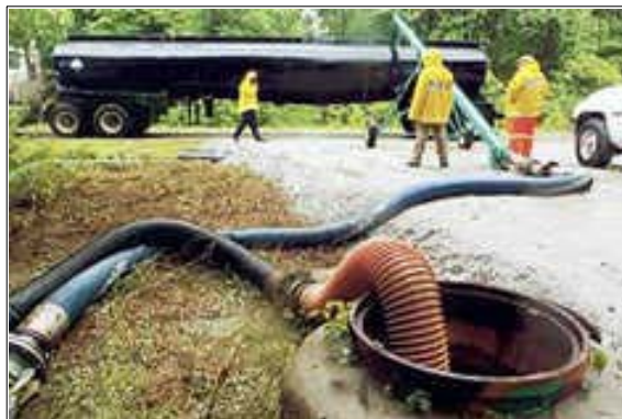
Town of Cary employees pump sewage from a manhole into a tanker truck along Lilly Atkins Road.
